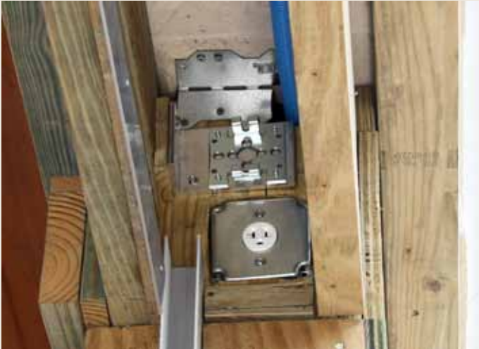
Unfinished cavity and column showing mounting brackets, electrical connections, and U-channel placement
